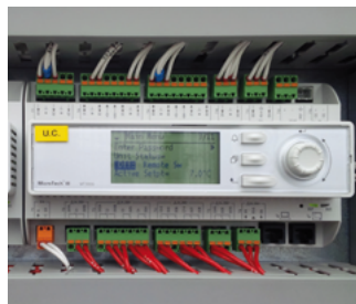
Controller box upgrade
